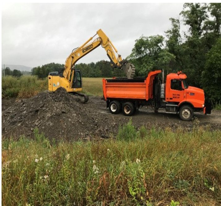
Above: Removal of sediment in the upper SVE high school sediment basin
